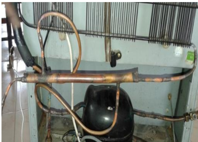
Fig.12. Heat Exchanger Fitted to the Refrigerator.
