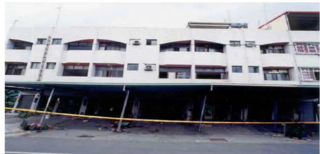
Fig.2.General mode of failure in OGS buildings.
